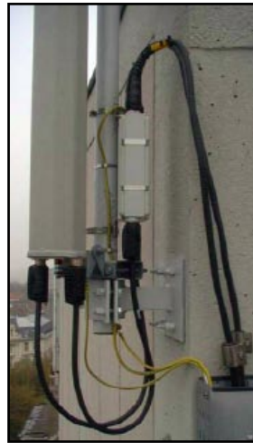
Figure 6: Site installation of a Stand Alone Antenna with separate TMA that would be enhanced by use of an Embedded LNA Antenna.
